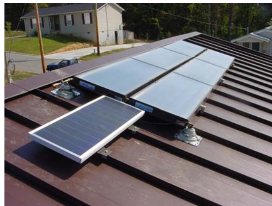
Figure 6. Solar water heater collectors.
